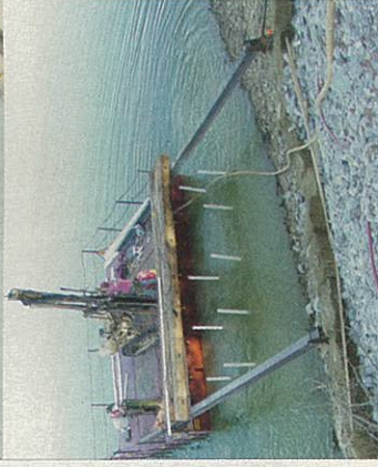
Top: A mini excavator, lowered into the shaft with the use of a crane, loads shot rock into a bucket.
